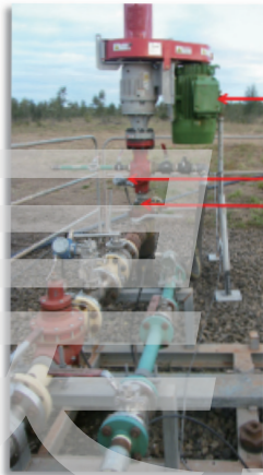
PCP Motor Electrical Gauge Outlet Fibre Optic DTS Outlet
